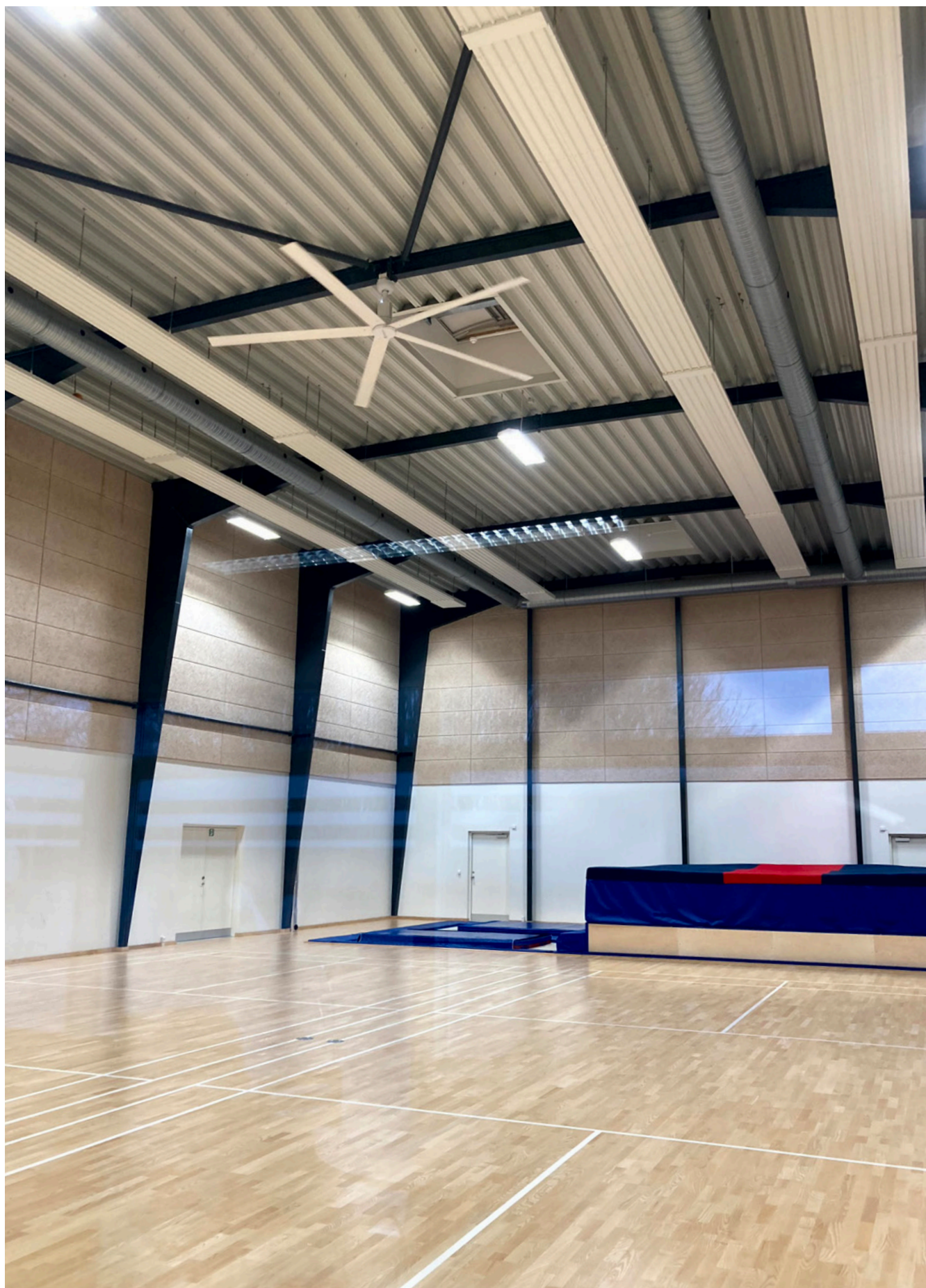
HVLS Ventilatorer, Alminde-Viuf Hallen
